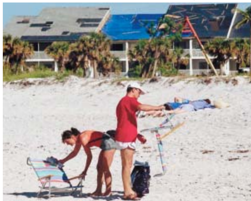
Bruce Bradley of York, Pa., had things in focus on Sanibel Island last week. On Captiva Island, Hurricane Charley cut a swath along Gulf Drive, and the damage to South Seas Resort, roofs and all, was huge.
